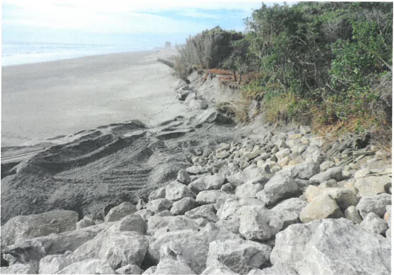
Northern end of wall showing seawall extension into dune face, underlying waste rubble (brown coloured rock) and 5 x large 'toe rocks' along erosion scarp 22 March 2016.
